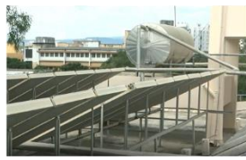
18 kW solar hot water system, Around 3000 ltr/day hot water
