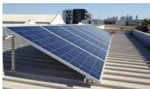
solar PV system
