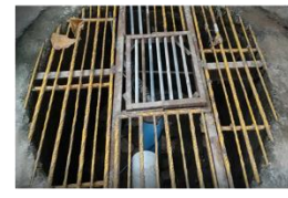
Rain Water Harvesting system capacity 4,20,000 ltrs
