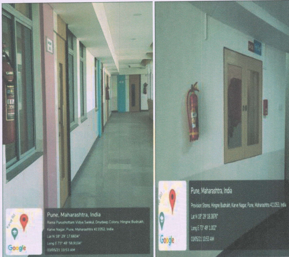
Fire Extinguishers and Fire Shaft in Corridor
