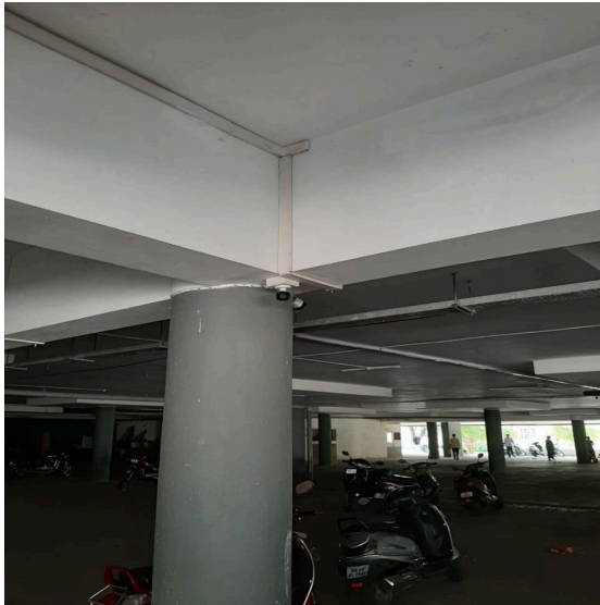
CCTV at Parking
