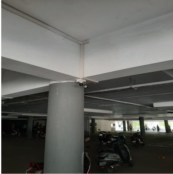
CCTV at Parking
